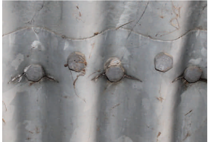
Bolt line cracking in newer CSP inspected by Keystone in 2012
