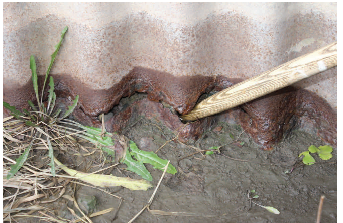
Perforation at mud line of 22 year old CSP inspected by Keystone in 2012
